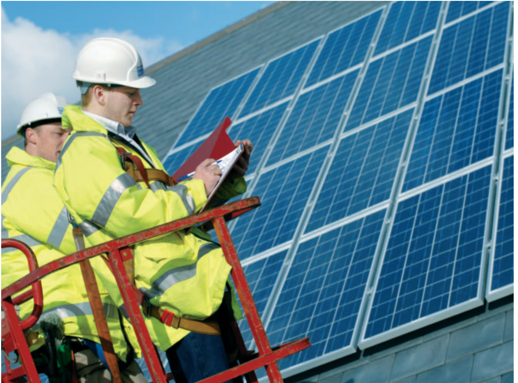
Photovoltaic cells, which convert solar light into electricity, cover an area of 30 sqm at the Cyan Building, Rotherham.
